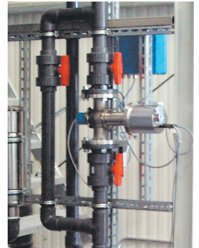
Straight pipe installation with ultrasonic cleaning system
